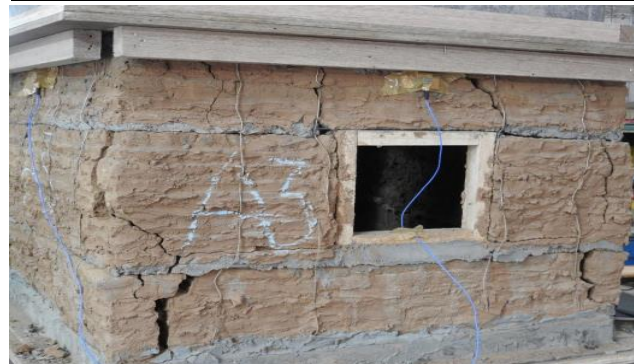
Figure 8: Failure of wall Junction and upper horizontal EQ.
