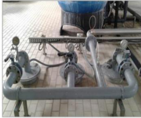
Picture 1: Centrifugal pumps of the well basin
