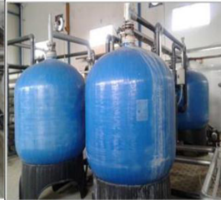
Picture 2: Sand filters
