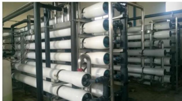
Picture 5: RO membranes in the treatment plant
